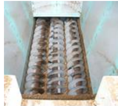
Mounting in discharge screw (wood-fired power plant)
