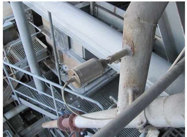
Mass flow meter MF3000 mounted on the conveying line of the aluminium oxide
